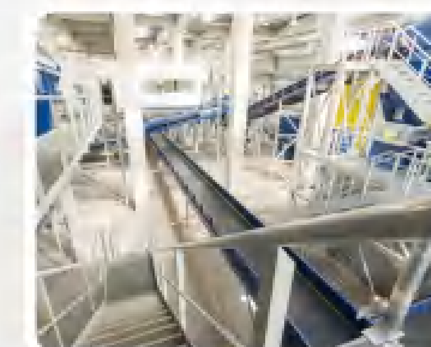
Total system visual monitoring
